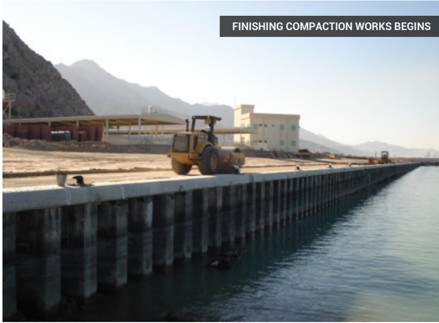
READY FINAL COMPACTION CONTINUES NOW THAT ALL SHEET PILES AND TIE RODS ARE INSTALLED
