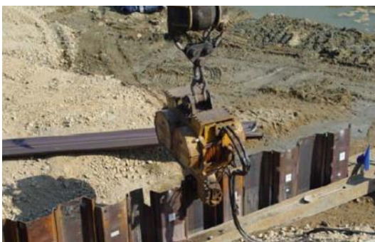
⑤ Drive the sheet piles after the drying the DPS-500 (after one day).
