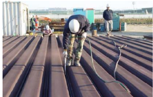
② Remove the dust or rust in the interlocks using an air compressor.
