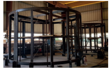
SEA WATER INTAKE PIPELINE RISE FISH CAGE
